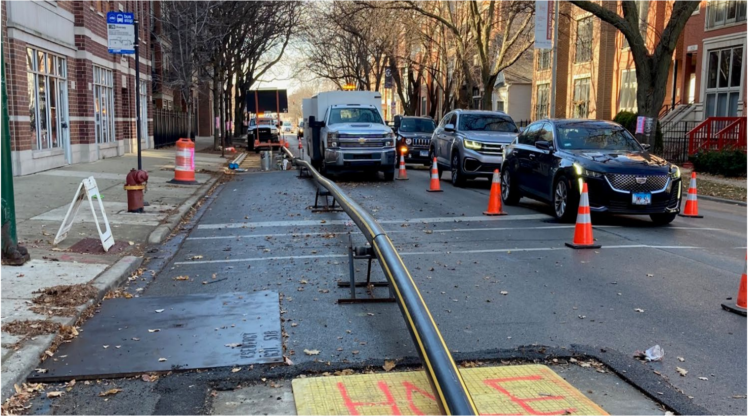
1700-2000 W. Diversey System Improvement Installation of 6" PLMP inserted into 12" CIMP Total of 2,138 of 6"PLMP installed.
